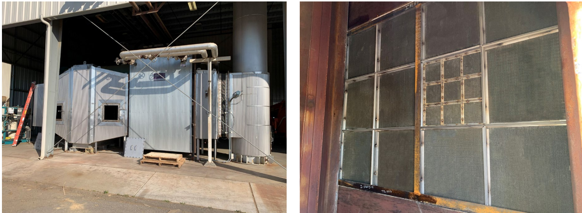
Figure 7: Package boiler with TripleCat DNX-LT installed upstream stack.
