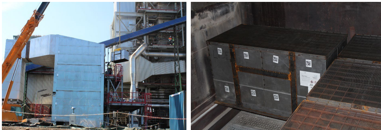
Figure 6: Pictures from the installation of TripleCat DNX-LT SCR catalyst at the biomass plant.
